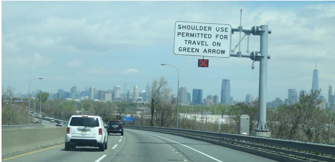
Figure 59. Photo. Mast Arm Dynamic Lane Control Sign, New Jersey Turnpike Newark Bay Extension.
